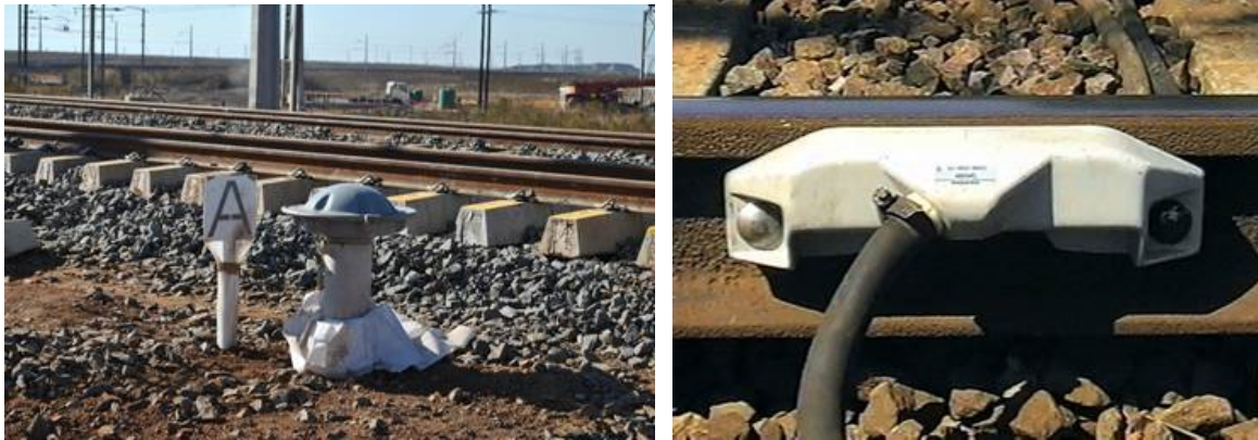
Figure 9 – Example of track vacancy detection equipment
